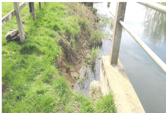
Photo 1 – Showing the Bridge Erosion
