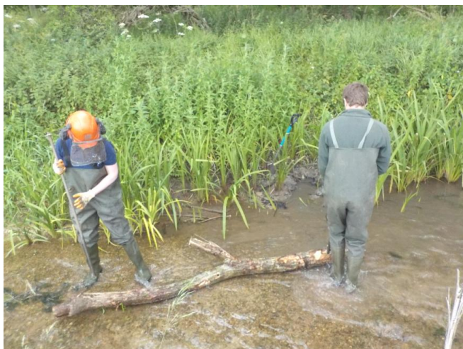
Photo: CWPT Ranger team using steel reinforcing bar to fix LWD in place on the Ampney Brook
